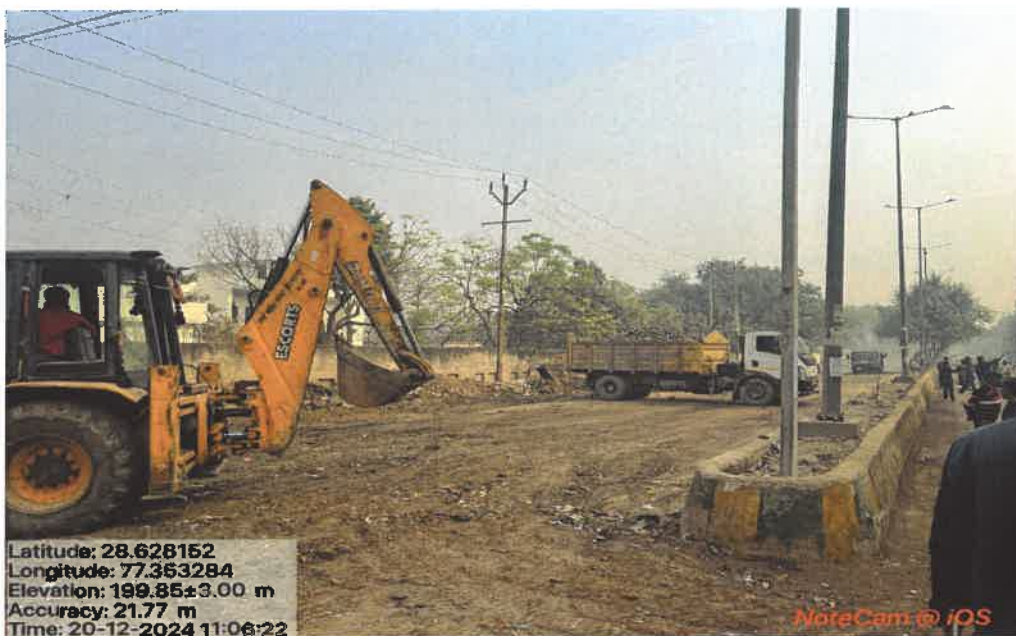
Figure 1: Site Photograph of Mixed Waste on Roads.
